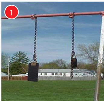
1 Swing chain should be unwrapped/inspected and broken swing seat should be replaced.
